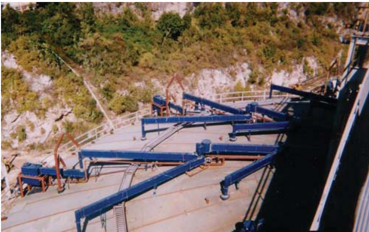
Distribution Air-Slides at top of Silo
